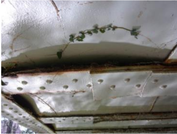
Above - Image 1: Plate deflection of transverse beams
