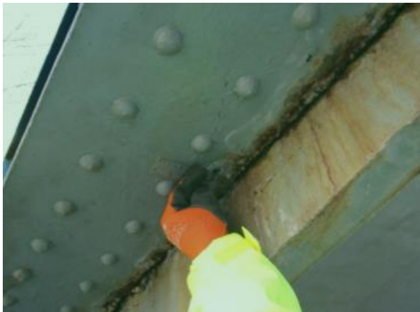
Above - Image 2: Corrosion of main edge girders
