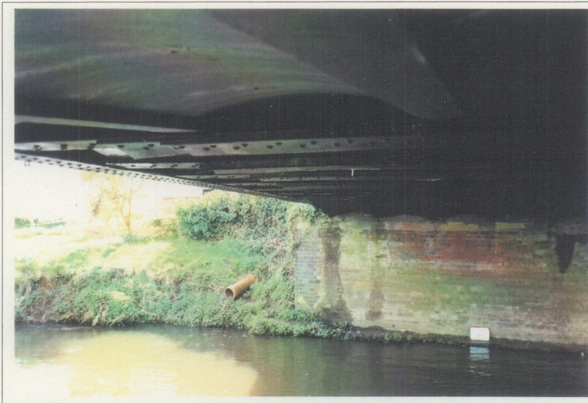
PLATE 7 DECK SOFFIT SHOWING DEFORMED FLANGE PLATES
