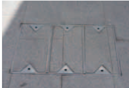
Paving pattern and bond aligned
