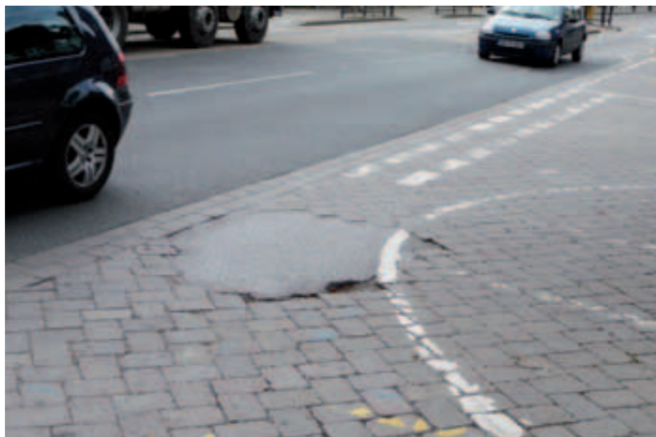
Poor reinstatement of block surface
